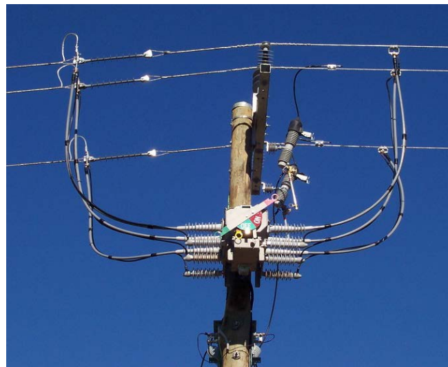
Figure 4-22 Load break switch/sectionaliser in the field
