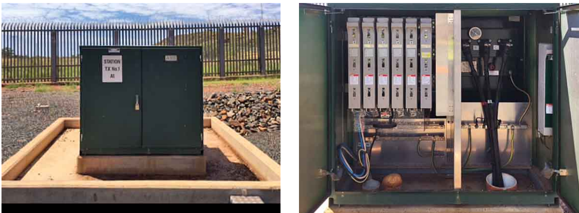
Figure 6-25 Typical substation transformer
