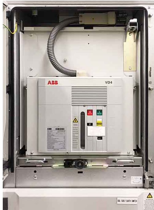
Figure 6-10 Indoor vacuum circuit breaker
