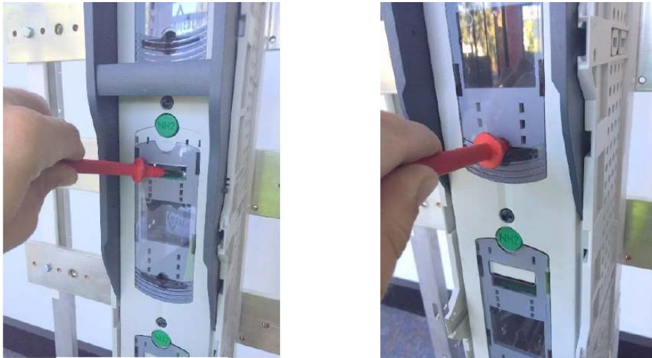
Figure 3-19: Testing busbar and cable side.
