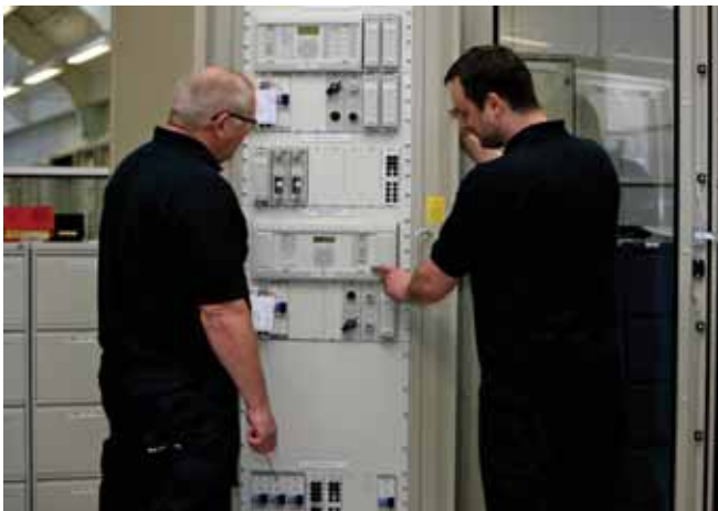
Factory acceptance testing
