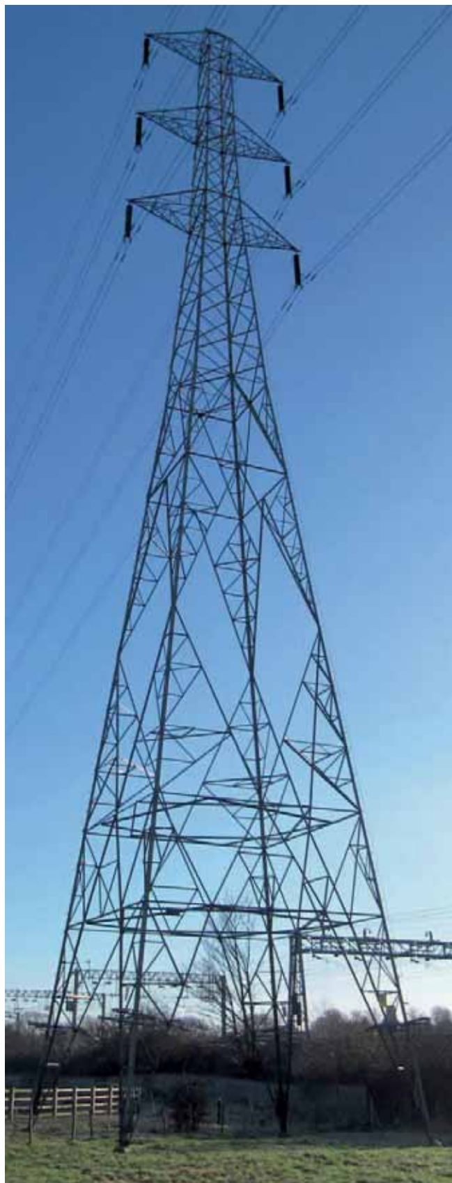
Figure 5.17: Double circuit 132kV overhead line tower
