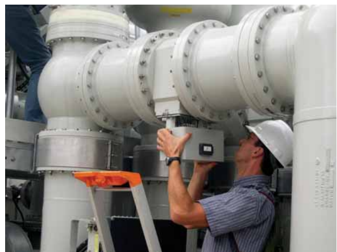
Figure 24.17: Rogowski coil installation in GIS
