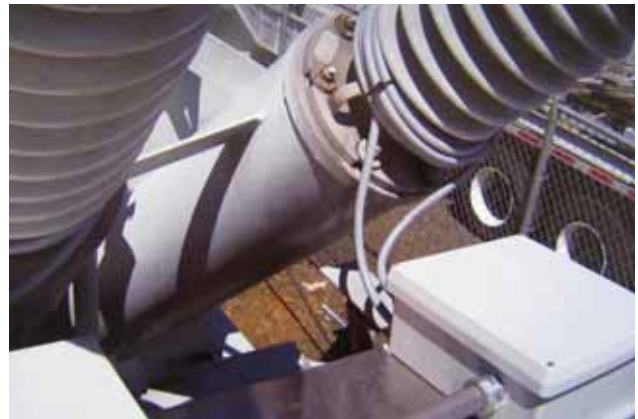
Figure 6.23: Alstom COSI-NXCT F3 flexible optical current transformer in a portable substation application
