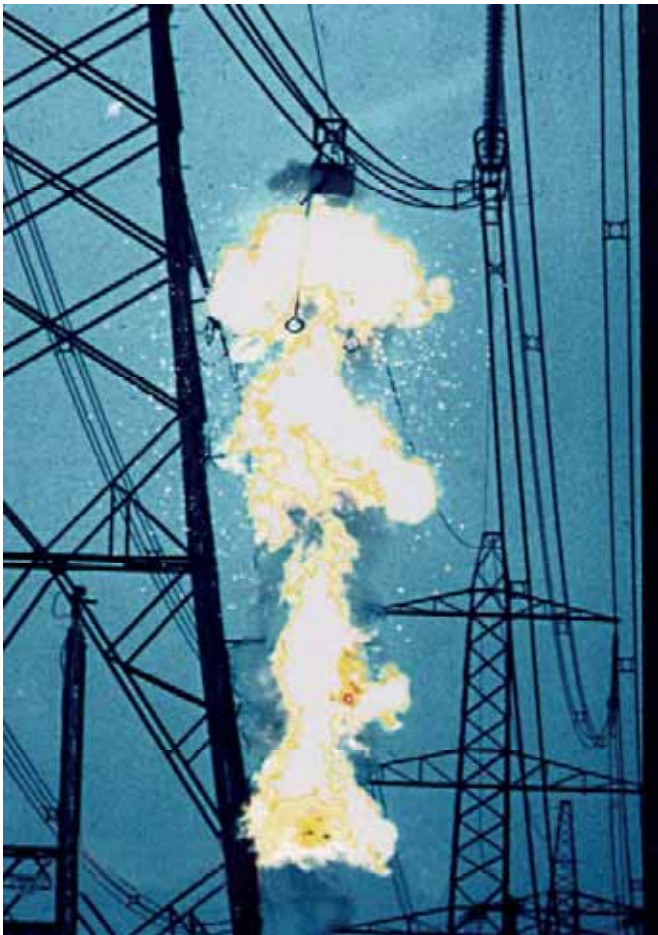
Figure 2.3: Onset of an overhead line fault
