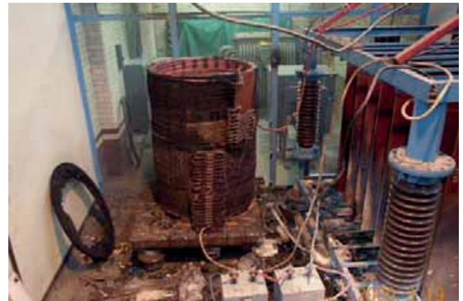
Figure 2.4: Possible consequence of inadequate protection
