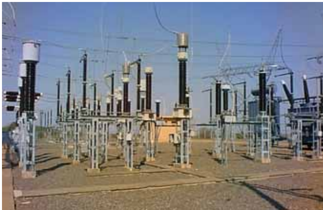
Figure 8.4: Carrier coupling equipment
