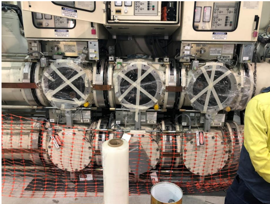
Figure 1: Parawebbing used to barrier out in service apparatus from accessible apparatus for GIS. Accessible gas points identified with yellow caps
