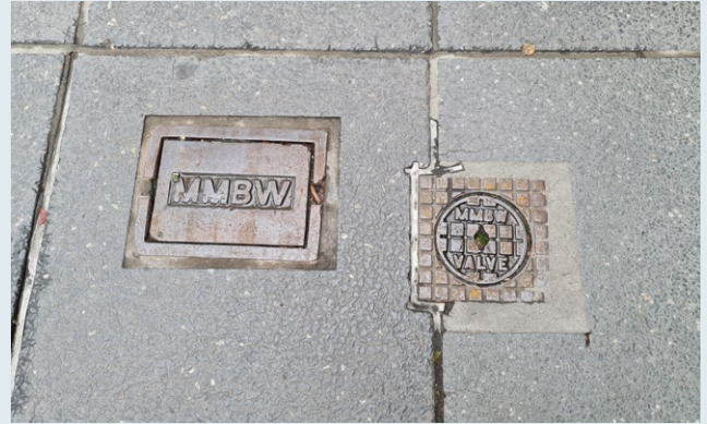
Figure 16: Hydrant connection points and water stop valves indicating water services underneath in close proximity.
