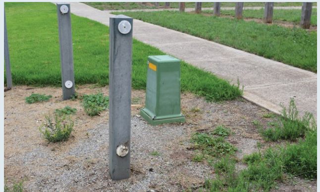
Figure 8: An underground pillar indicating low voltage electrical underground cables owned by the power company installed on public land.
