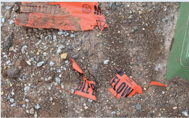
Figure 21: Orange marker tape to provide warning of underground electrical services.
