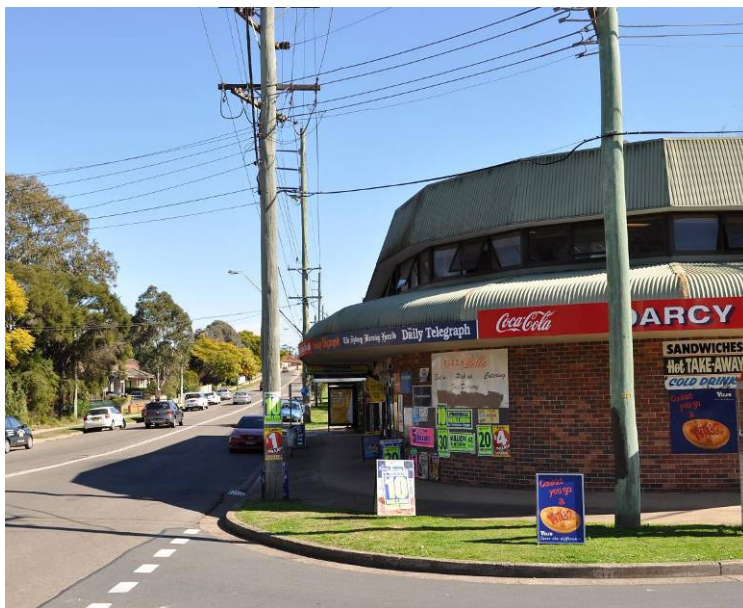
High and low voltage overhead mains
