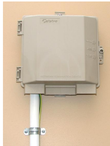
Cables hidden by the cover
