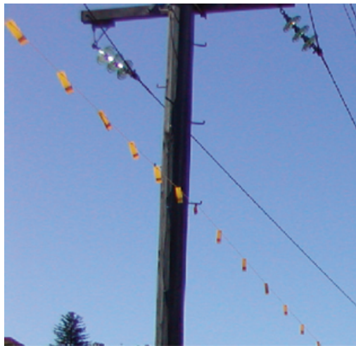
Figure 7: Illustration of a visual tape bunting fitted under overhead power lines.
