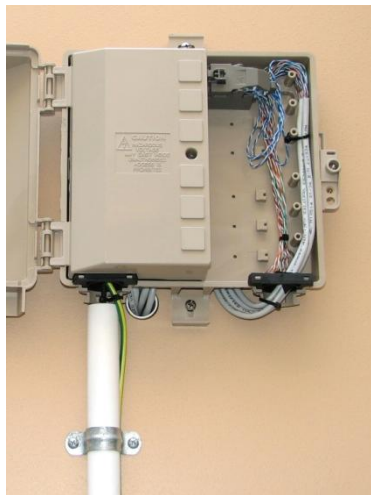
Cables running behind the NTD
