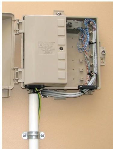
Cables running below the NTD
