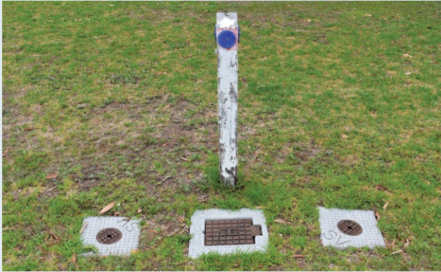
Figure 15: Hydrant connection points and water stop valves indicating water services underneath in close proximity.
