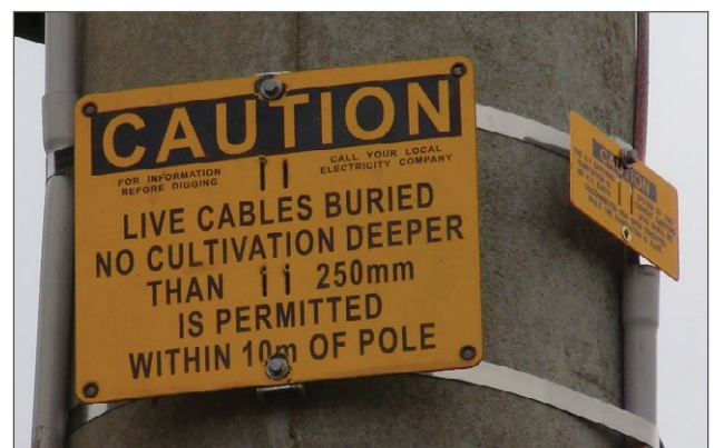
Figure 27: Example of warning signage installed on a pole
