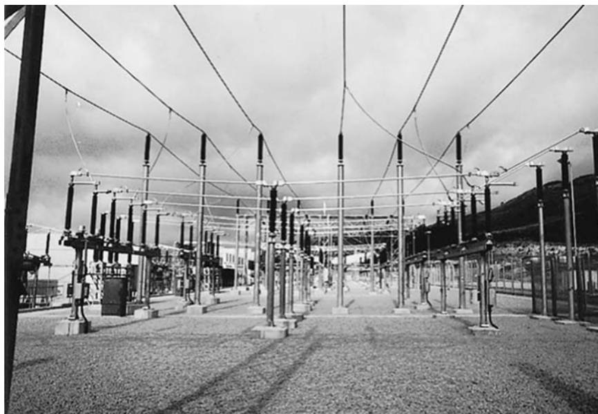
Figure 18.16 'Tarantula' 132 kV busbar
