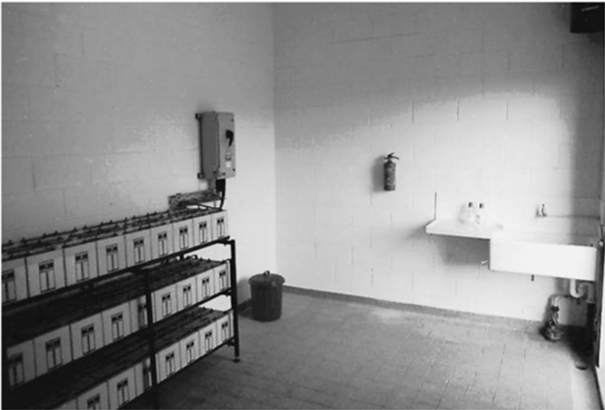
Figure 4.3 Primary substation battery room DC distribution and charger (courtesy of Balfour Beatty Projects and Engineering Ltd)
