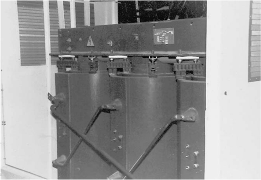
Figure 14.24 1 MVA, 21/0.4 kV, cast resin transformer
