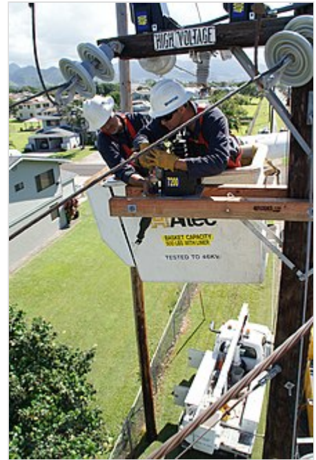
Working under tension from an electrically insulating platform in a medium voltage network
