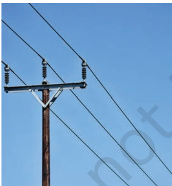
Fig. 4.54 Low Tension Distribution Lines (LT)
