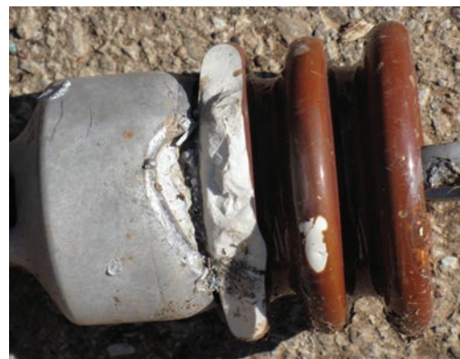
Fig. 4.65 Wire Insulation Damage
