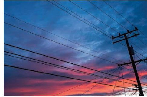
Fig. 4.50 Power Distribution Lines
