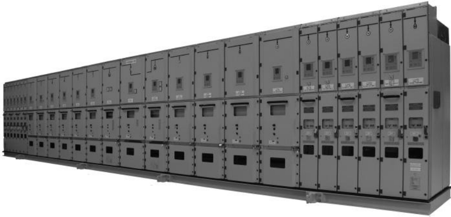
Figure 6.1 A typical ABB UniGear type ZS1® (courtesy of ABB). MV, arc-proof, air-insulated, metal-clad switchgear11.
