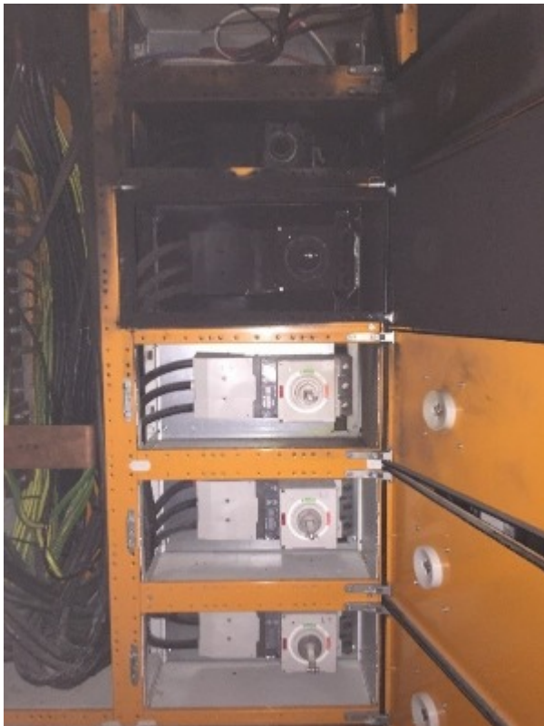
Damage caused by the arc flash explosion.
