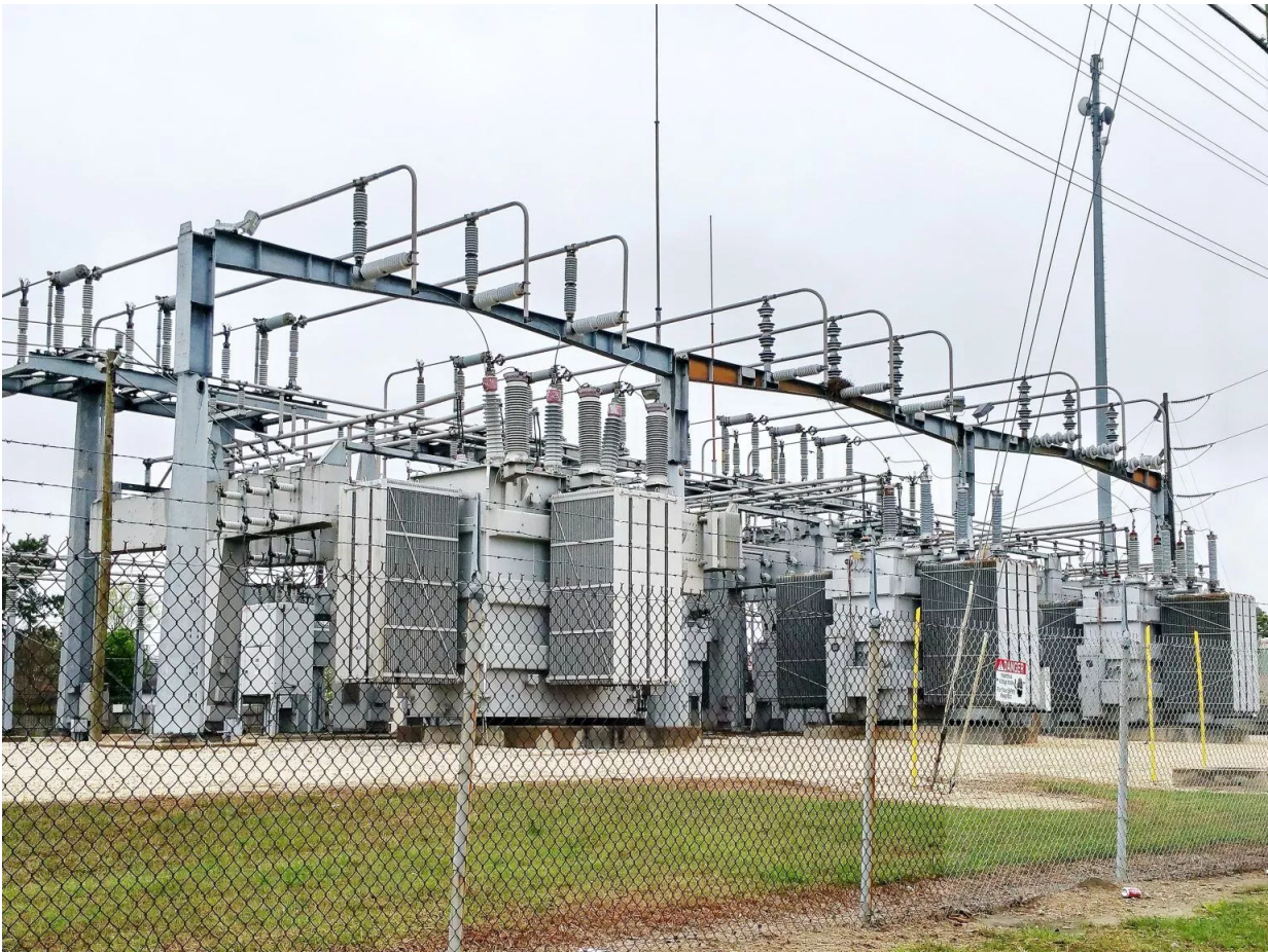
Figure 1(a) Substation Photo by ETA+ on Unsplash
