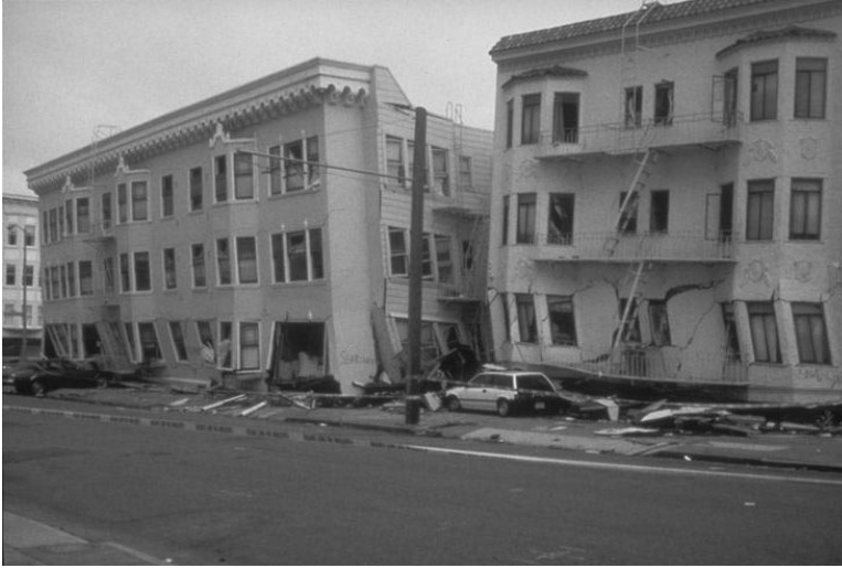
FIGURE 18.37 Soft story collapse in San Francisco during the 1989 Loma Prieta Earthquake. (Photo courtesy of the USGS; The Loma Prieta , USGS, 1998.)
