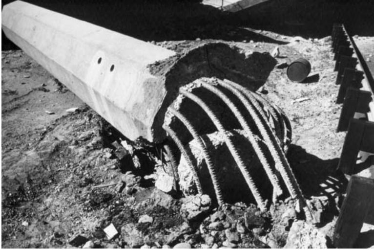
FIGURE 18.35 Failure of column to pile shaft connection.
