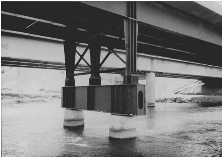
FIGURE 18.86 Lead-rubber isolation bearings on the All American Canal Bridge in California.
