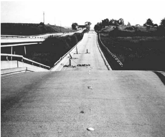
FIGURE 18.26 Piles penetrating bridge deck.
