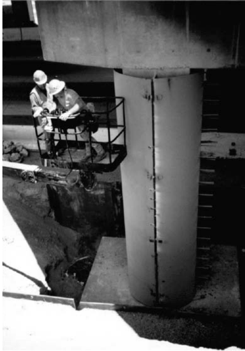
FIGURE 18.89 Steel shell being wrapped around a concrete bridge column to increase its ductility and shear strength.
