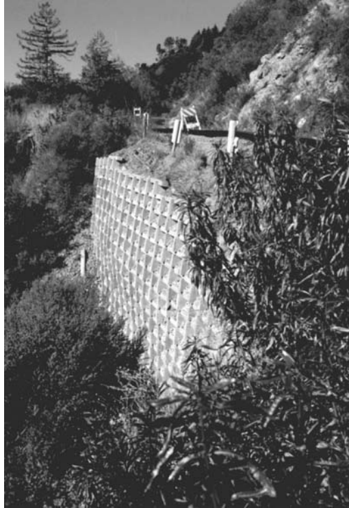
FIGURE 18.74 Crib wall continues to support steeply sloping soil in Santa Cruz after the 1989 Loma Prieta Earthquake. (Photo courtesy of EERI.)
