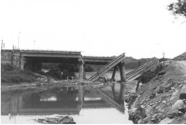
FIGURE 18.19 Collapse of Tsu Wei Bridge due to landslide during the Ji Ji, Taiwan, earthquake.
