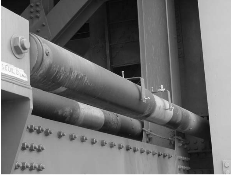
FIGURE 18.88 The Vincent Thomas Bridge retrofit provided gaps between the decks and the towers and also fluid viscous dampers to dissipate energy. (Photo courtesy of Enidine Inc.)
