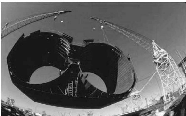
FIGURE 28.10 Steel immersed tunnel — Ted Williams Tunnel, Boston, MA (© David Sailors 1993, with permission).
