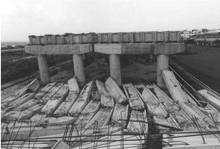
FIGURE 18.63 Collapsed precast, prestressed “I” girders during construction of new expressway in Taiwan due to the 1999 Ji Ji, Taiwan, earthquake.
