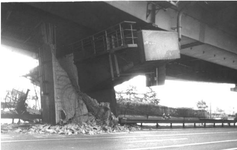
FIGURE 18.51 Shear failure of Pier 150 on Kobe Route 3.
