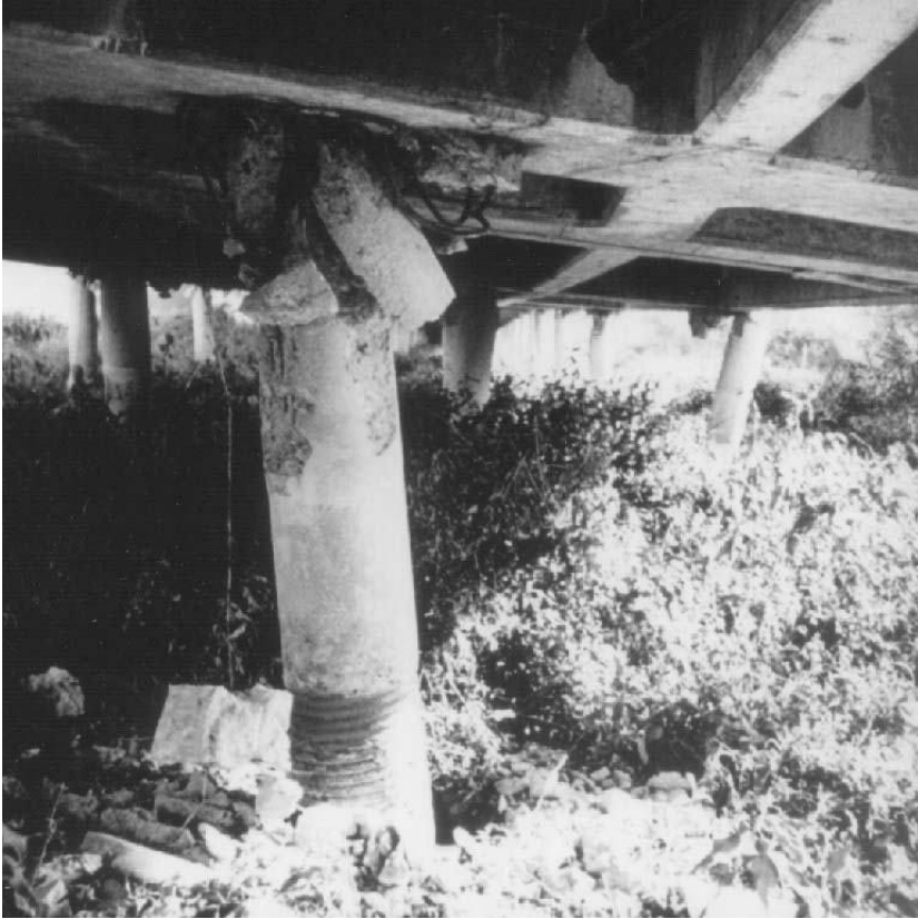
FIGURE 18.25 Broken piles under bridge.
