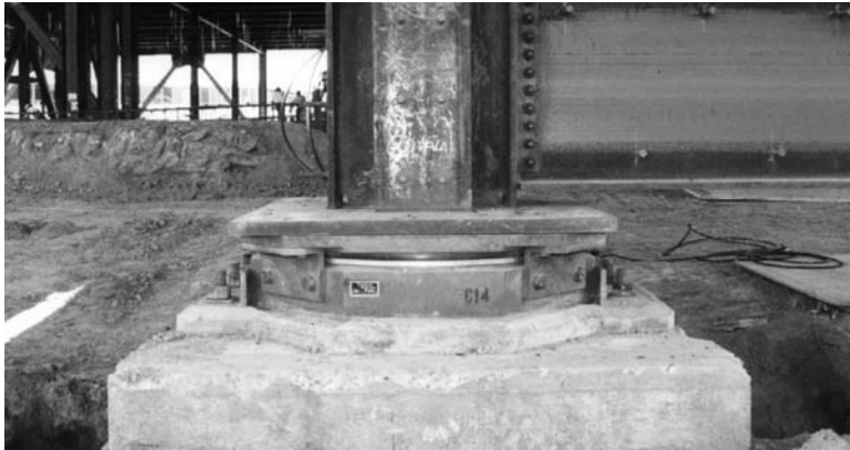
FIGURE 18.79 One of the 267 friction pendulum devices for the new San Francisco Airport International Terminal. (Photo courtesy of Earthquake Protection Systems Inc.)
