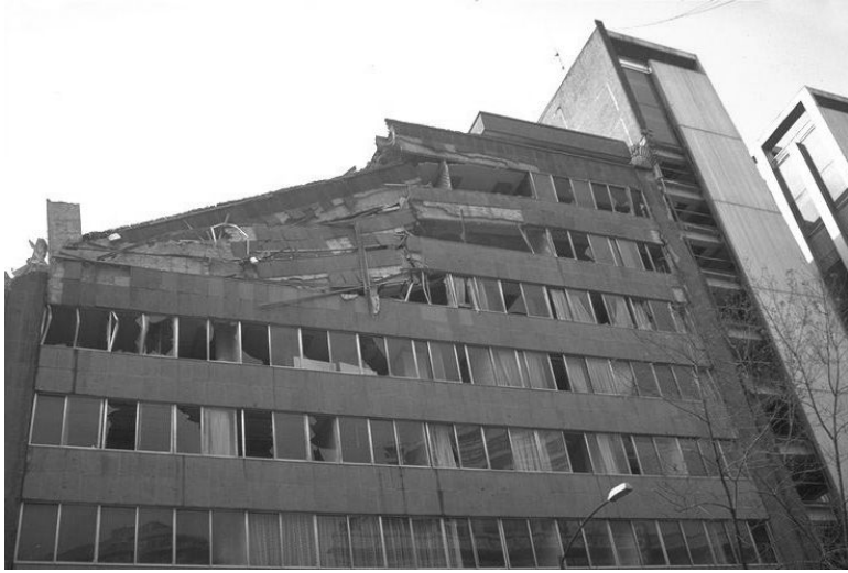
FIGURE 18.31 Damaged 10-story building between the Plaza de la Constitution and Zona Rosa in Mexico City. (Photo by Karl Steinbrugge, from the EERC NISEE Photo Library.)
