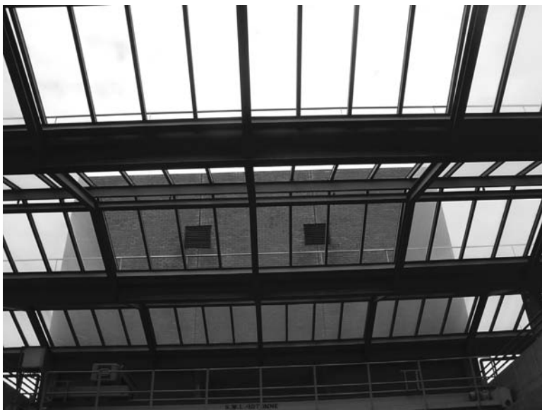
FIGURE 29.8 Broken glass panel due to thermal stress.
