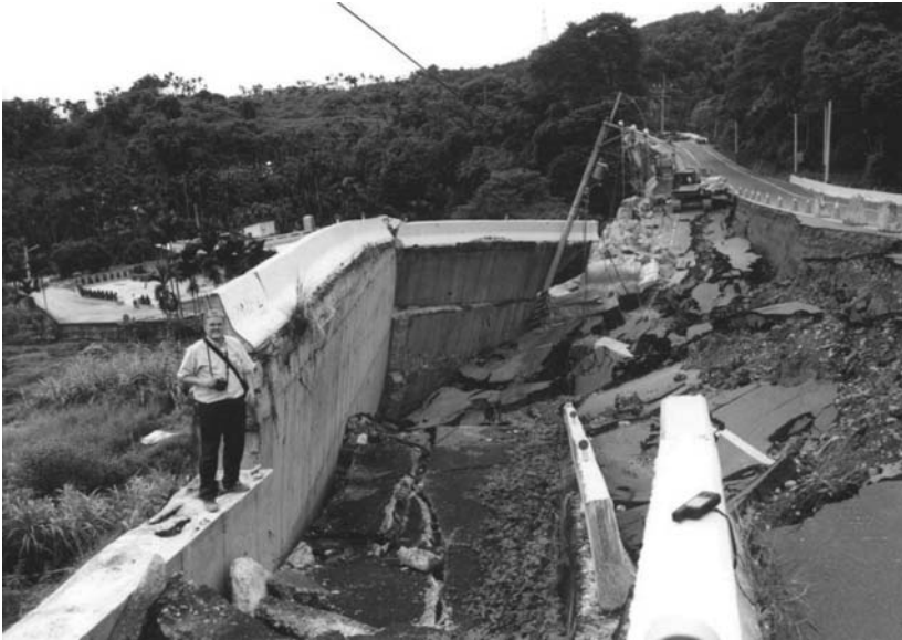
FIGURE 18.13 Gravity retaining wall pushed outward by landslide.
