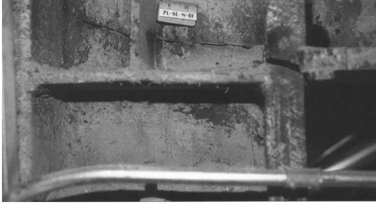
FIGURE 18.60 Steel moment-resisting frame connection after the 1994 Northridge Earthquake. (Photo courtesy of EQE International; EQE, EQE Int. Rev. , Fall, 1–6, 1994.)
