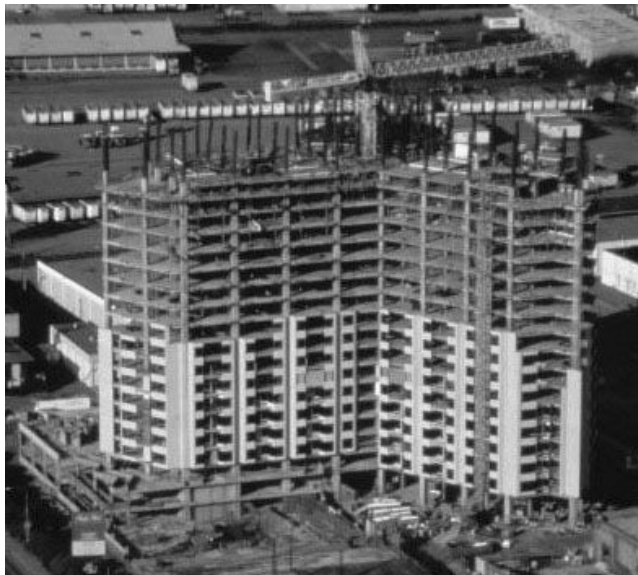
PHOTO 7.1 A 30-story reinforced concrete building under construction. The Pacific Park Plaza is one of the largest reinforced concrete structures in the San Francisco Bay area. It survived the October 17, 1989, Loma Prieta earthquake without damage. Instrumentation in the building recorded peak horizontal accelerations of 0.22g at the base and 0.39g at the top of the building (courtesy of Mr. James Tai, T.Y. International, San Francisco).
