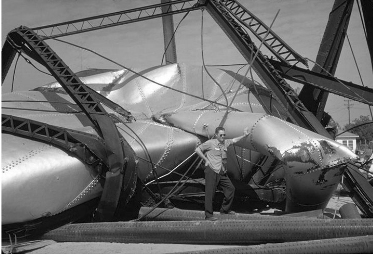
FIGURE 18.62 California Water Service 150,000-gal tank on six legs; the typical failure of tanks is upside down, with riser on top (Bakersfield, California, photo by Karl V. Steinbrugge, Steinbrugge Collection, slide/image No. S64, photo date July 25, 1952, Kern County, California, earthquake, July 21, 1952, magnitude 7.69; courtesy of Steinbrugge Collection, Earthquake Engineering Research Center, University of California, Berkeley).
