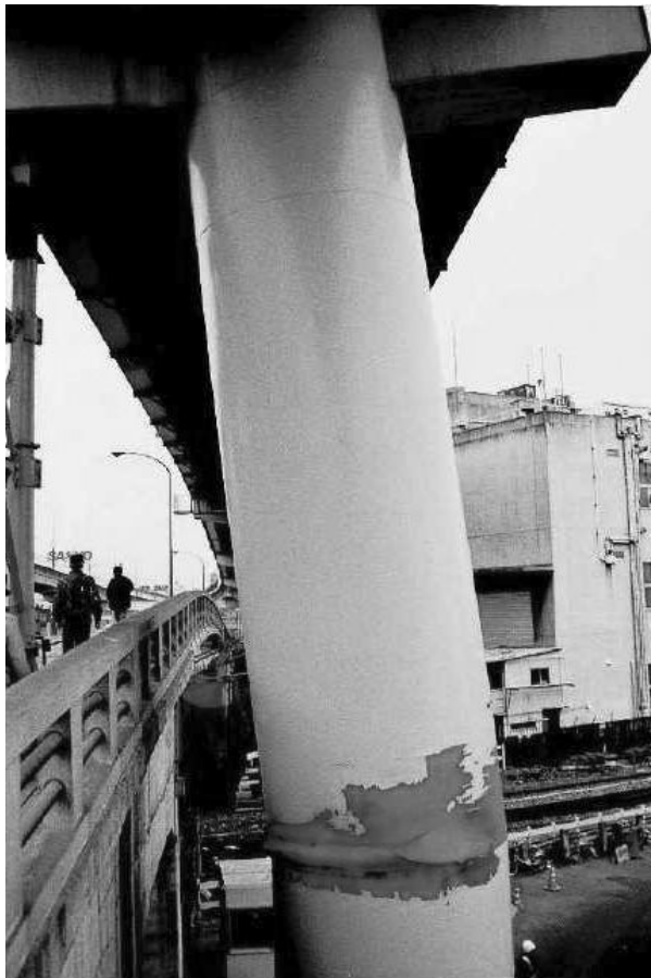
FIGURE 18.54 Pier 585 on Kobe Route 3 during the 1995 Kobe Earthquake. (Photo courtesy of Hanshin Expressway Public Corporation.)
