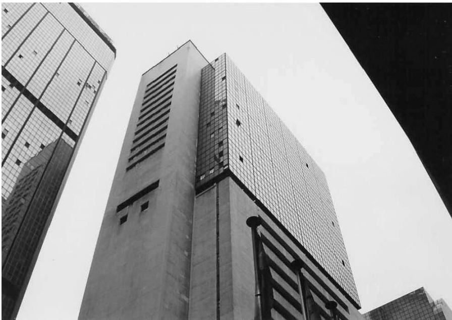
FIGURE 29.3 Damage of buildings after a typhoon attack.
