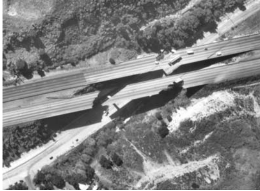
FIGURE 18.43 Damage to Gavin Canyon UC during the 1995 Northridge Earthquake.
