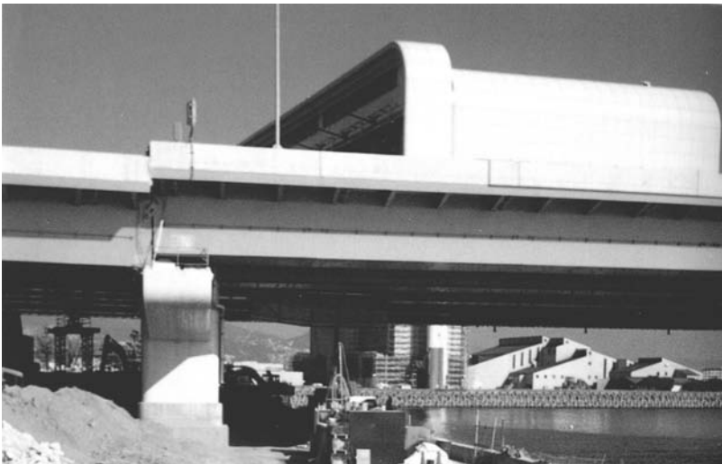
FIGURE 18.7 Liquefaction caused bridge damage during the Kobe Earthquake.
