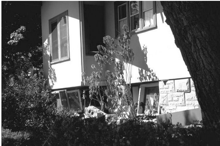
FIGURE 18.32 Failed hollow concrete block foundation during the magnitude 6.0, 1987 Whittier, California, earthquake. (Photo by Karl Steinbrugge. Photo courtesy of Steinbrugge Collection, Earthquake Engineering Research Center, University of California, Berkeley.)
