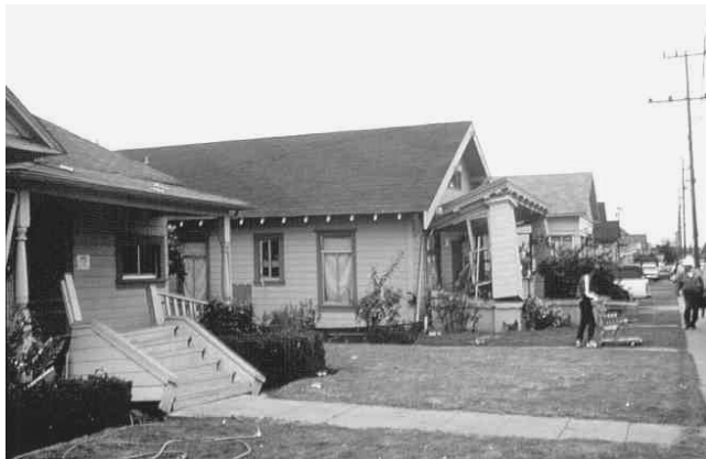
FIGURE 10.5 Houses damaged due to cripple wall failure, 1983 Coalinga Earthquake (courtesy of EQE International).
