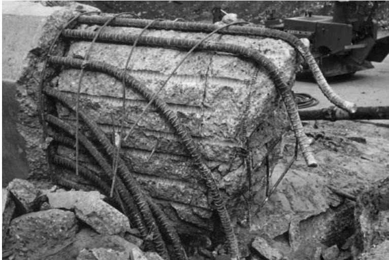
FIGURE 18.36 Failure of column to footing connection.
