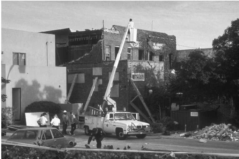
FIGURE 18.61 Rear view of damaged unreinforced masonry (URM) building facing Pacific Garden Mall, Santa Cruz Area, California. (Photo by James R. Blacklock, Loma Prieta Collection, Earthquake Engineering Research Center, University of California, Berkeley.)
