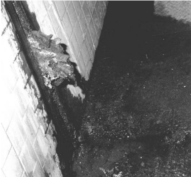
FIGURE 18.11 Liquefaction induced damage to the Webster Street Tube tunnel.
