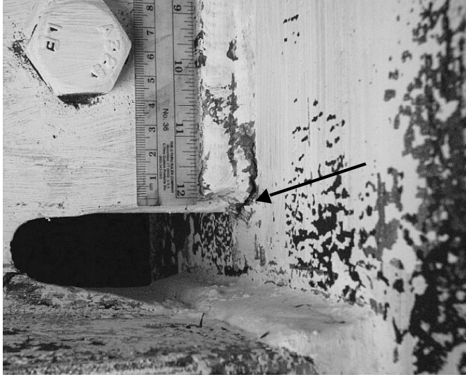
FIGURE 34.8 Low-cycle fatigue crack developing at the end of the beam web to column flange weld in a moment-frame connection.
