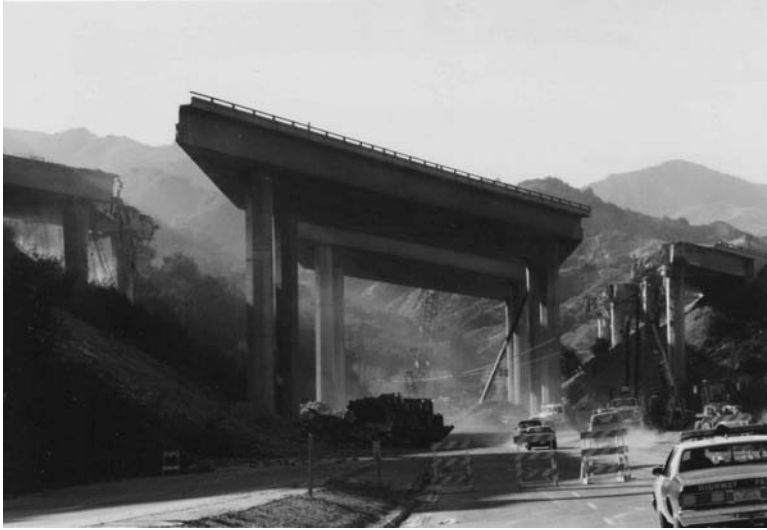
FIGURE 20.2 Collapse of I-5 Gavin Canyon Undercrossing, California, in the 1994 Northridge Earthquake.
