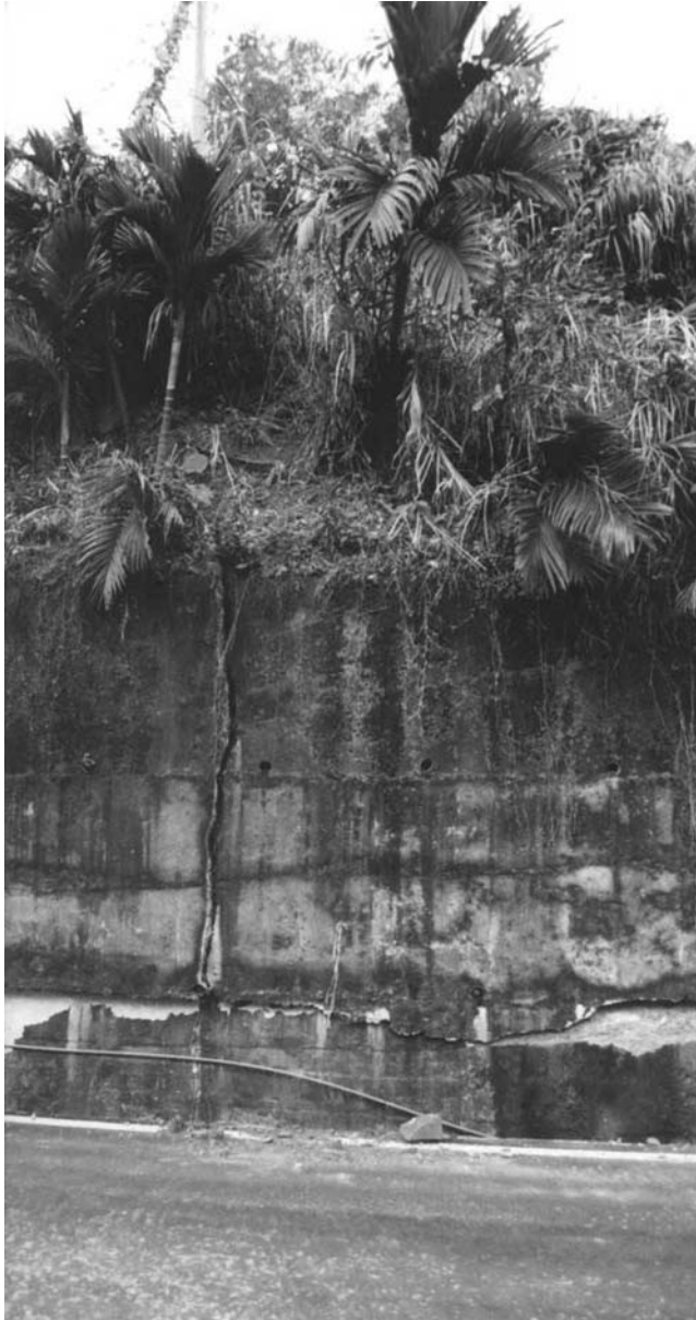
FIGURE 18.14 Gravity retaining wall with shear damage from landslide.
