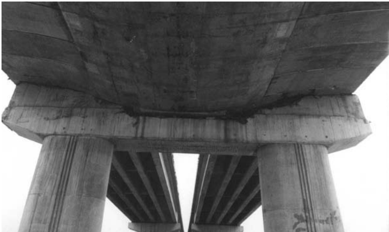
FIGURE 18.45 Damage at end-supports to Ji Lu cable-stayed bridge.
