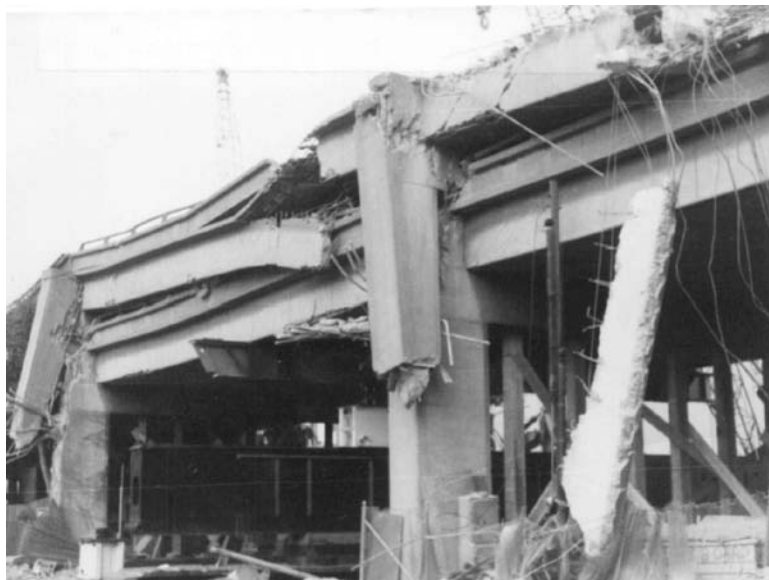
FIGURE 18.28 Damage to Cypress Street Viaduct.
