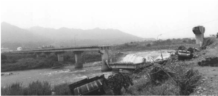
FIGURE 18.67 The Dajia River bridge and 6-m fault scarp.
