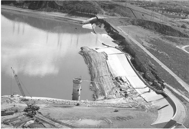
FIGURE 18.21 Damage to the Lower San Fernando Dam. (Photograph courtesy of Steinbrugge Collection, Earthquake Engineering Research Center, University of California, Berkeley.)
