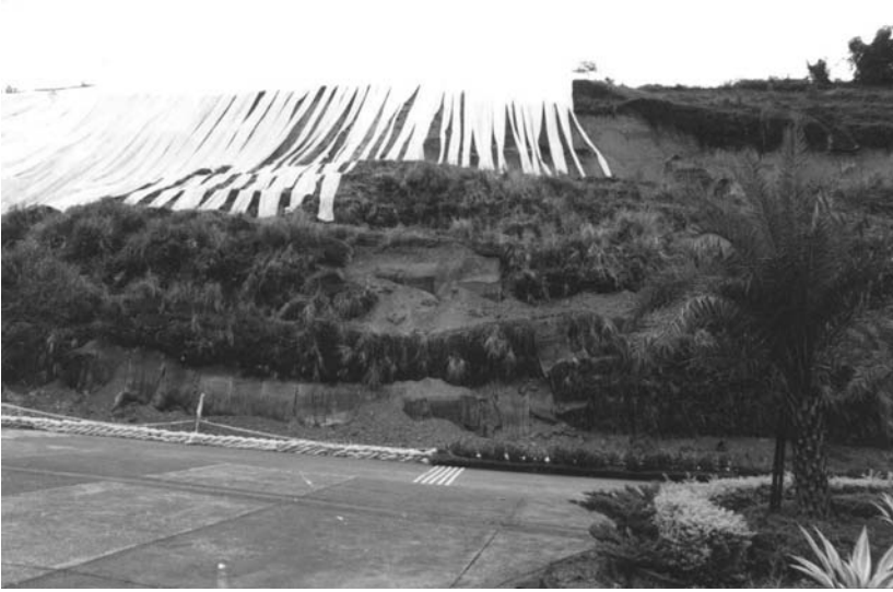
FIGURE 18.15 Fabric retaining wall damaged during the 1999 Ji Ji, Taiwan, earthquake.
