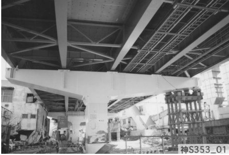
FIGURE 18.68 Collapsed building leaning against the Kobe Route 3 Expressway. (Photo courtesy of Hanshin Expressway Public Corporation.)
