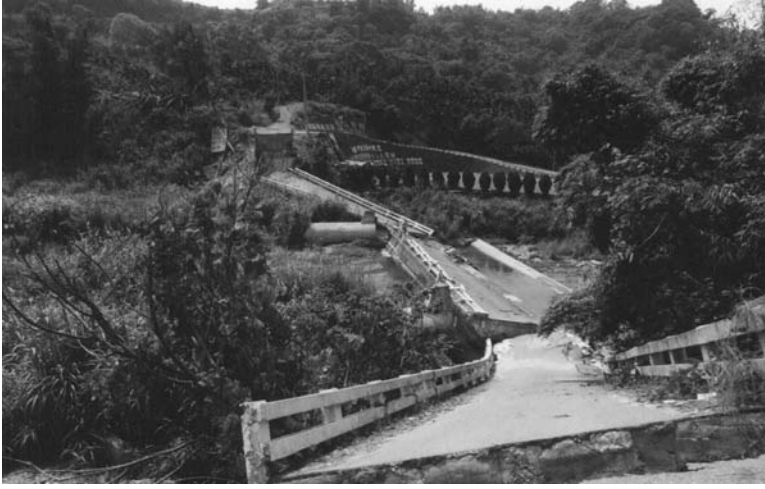
FIGURE 18.33 Three-span bridge rocked over during the 1999 Ji Ji, Taiwan, earthquake.
