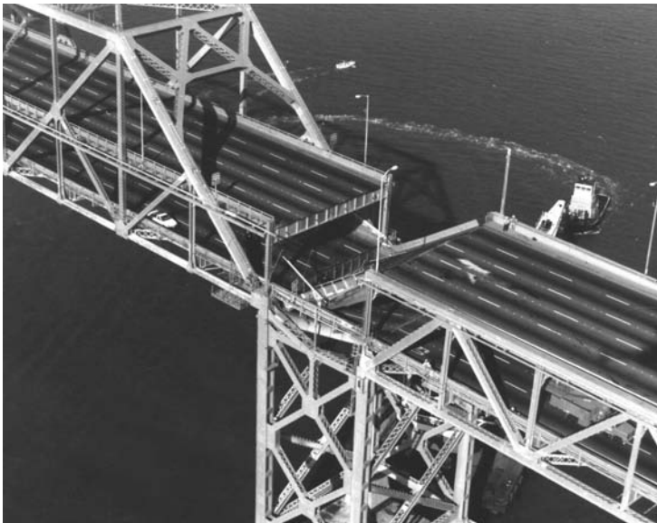
FIGURE 20.1 Collapse of eastern portion of San Francisco-Oakland Bay Bridge in the Loma Prieta Earthquake (courtesy of California Department of Transportation).
