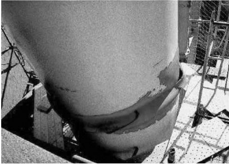
FIGURE 18.55 Torn buckle of steel column on Route 3 after the 1995 Kobe Earthquake. (Photo courtesy of Hanshin Expressway Public Corporation.)
