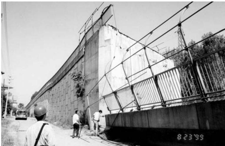
FIGURE 18.73 Mechanically stabilized earth wall continues to support the embankment behind the collapsed Arifiye Overcrossing after the 1999 Kocaeli, Turkey, earthquake.
