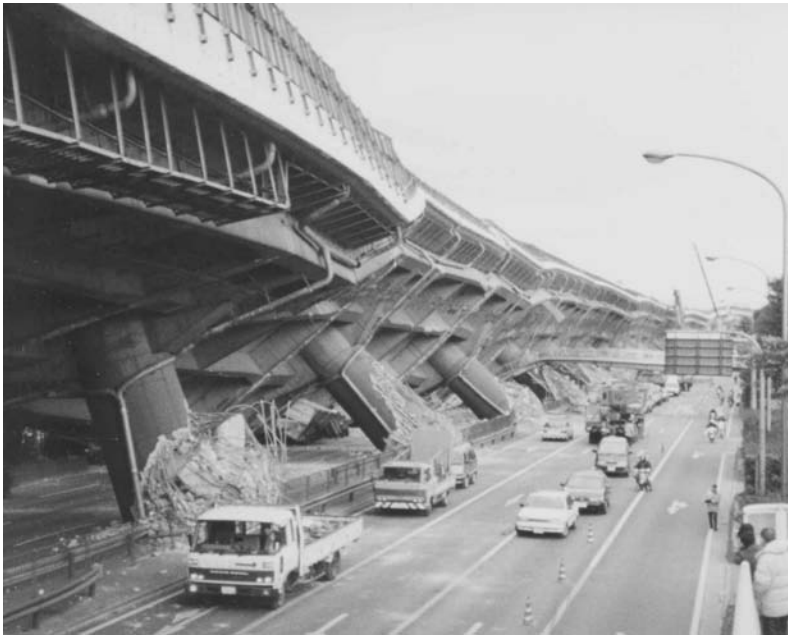
FIGURE 20.3 Collapse of Hanshin Expressway in the 1995 Hyogo-Ken Nanbu Earthquake in Japan (courtesy of Mark Yashinsky).
