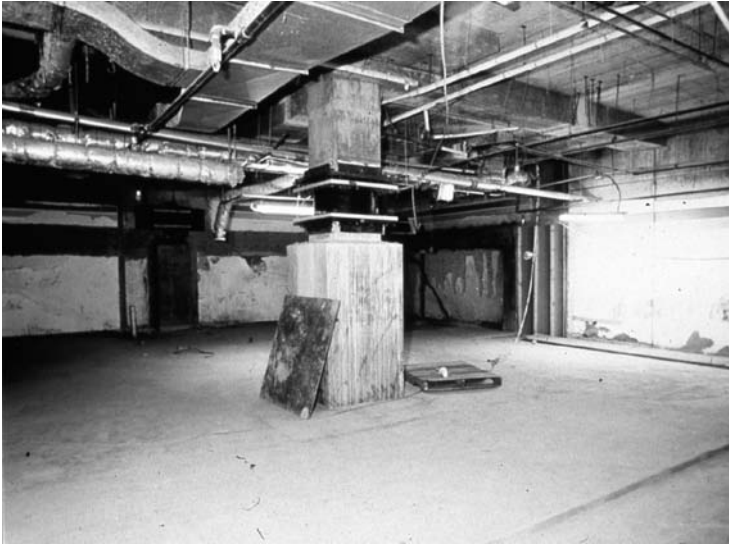
FIGURE 18.85 The concrete columns were cut at midheight and lead-rubber isolation devices were installed. (Photo courtesy of Dynamic Isolation Systems Inc.)
