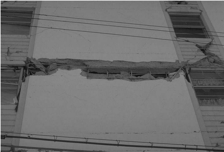
FIGURE 18.49 Damage to north side of Mt. McKinley Apartments. (Photograph by Karl Steinbrugge, Earthquake Engineering Research Center, University of California, Berkeley.)
