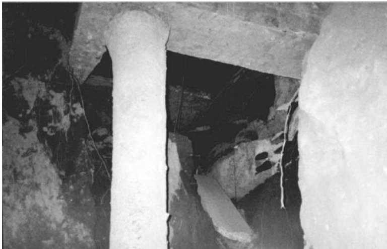
FIGURE 18.69 Washed-out abutment fill caused by water pipe break.
