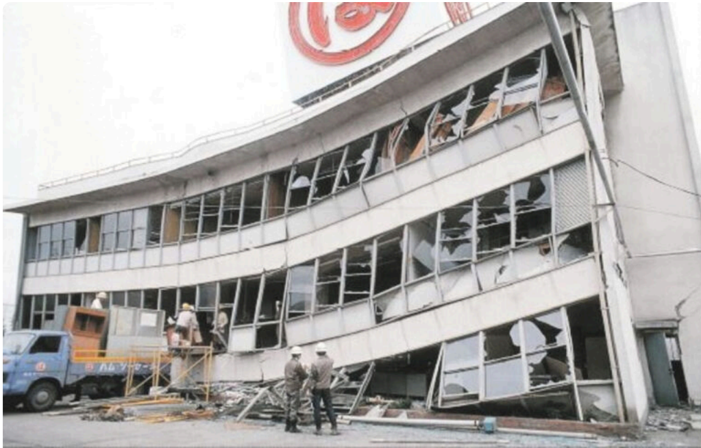
Damage from the 1978 Miyagi Earthquake: Collapsed Building in Sendai
