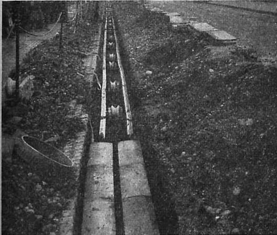
FIG. 79. CABLES IN TRENCH PROTECTED BY CONCRETE COVERS
