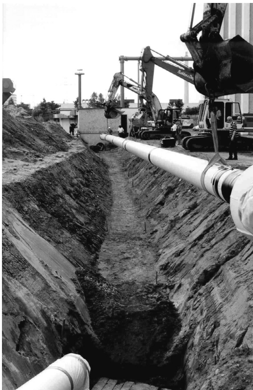
FIGURE 18.20 Trench of 55-m-long section during laying and view into the trench. (Courtesy of Siemens.)
