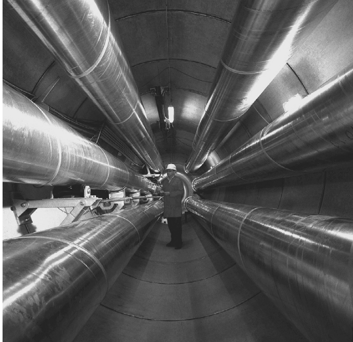
FIGURE 18.15 Tunnel arrangement of two systems GIL for the long-term test. (Courtesy of Siemens.)
