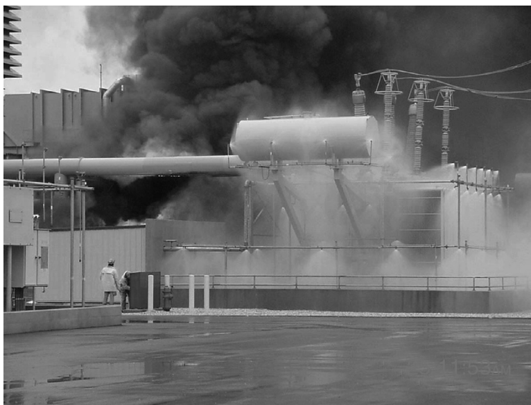
FIGURE 14.1 Shows a transformer deluge system in operation during a fire.
