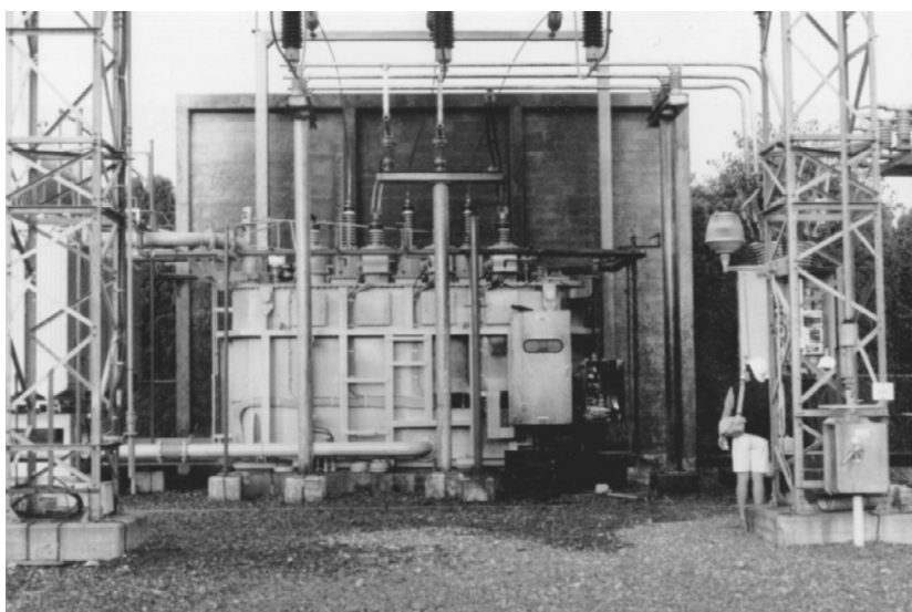
FIGURE 14.2 Shows the aftermath of a transformer fire where deluge water spray and a fire wall were in place.
