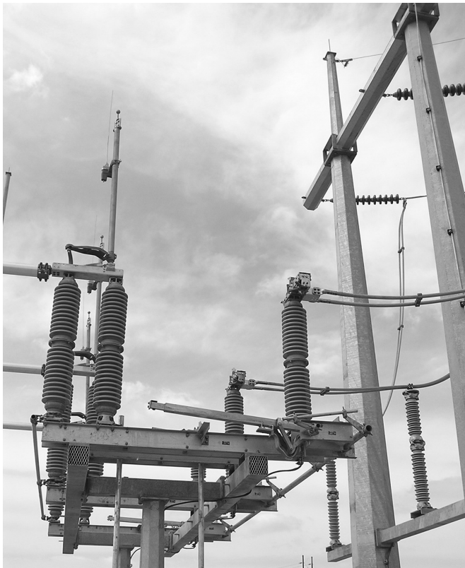
FIGURE 4.24 Grounding switch integrally attached to vertical break disconnect switch.
