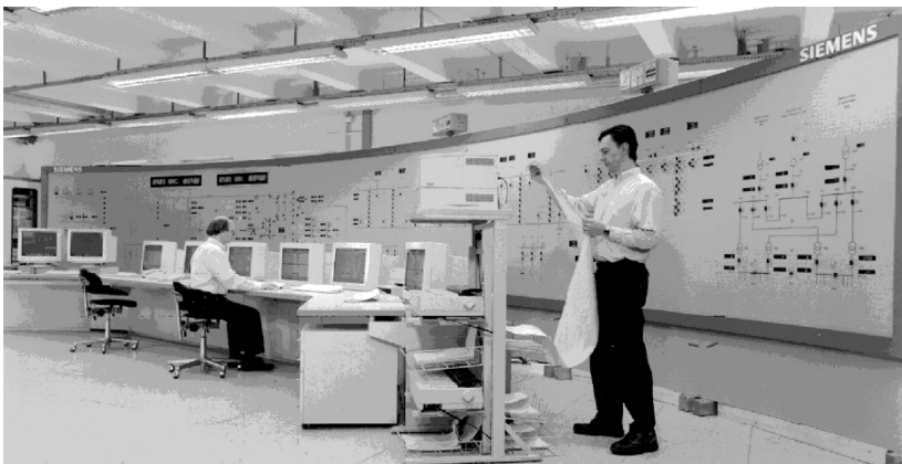
FIGURE 5.21 Controls for a \pm 500 kV, 1800 MW HVDC; function test. (Photo courtesy of Siemens.)
