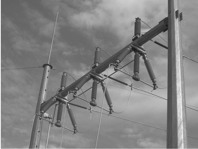
FIGURE 4.10 Underhung mounted disconnect switch.
