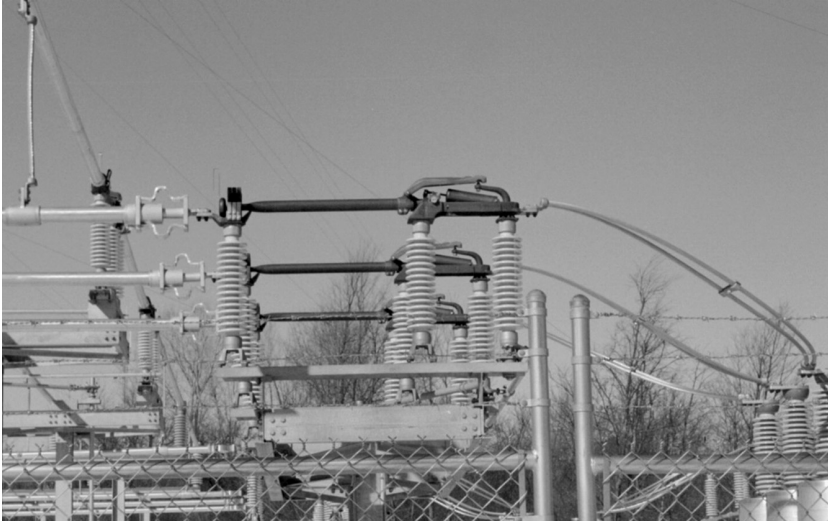
FIGURE 4.8 Horizontally upright mounted disconnect switch.
