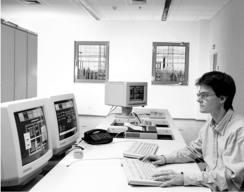
FIGURE 5.20 Local control desk of a 600 MW back-to-back converter station. (Photo courtesy of Siemens.)
