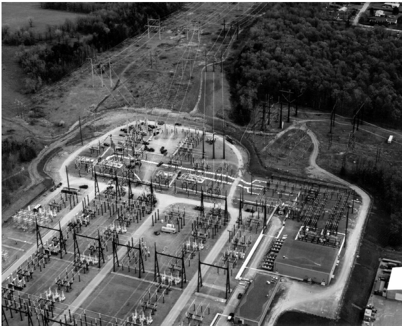
FIGURE 5.18 Convertible static compensator (CSC) at NYPA's 345 kV Marcy, New York substation. (Photo courtesy of New York Power Authority.)
