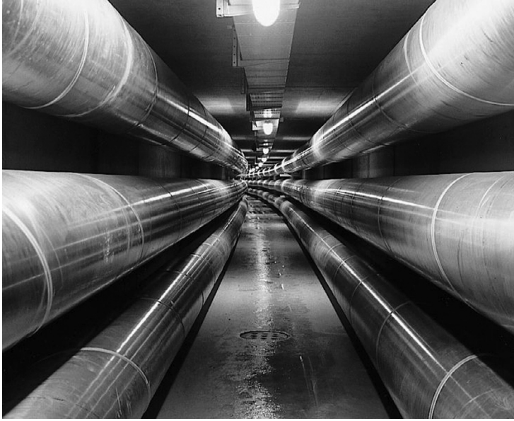
FIGURE 18.8 Tunnel-laid GIL for voltages up to 550 kV. (Courtesy of Siemens.)
