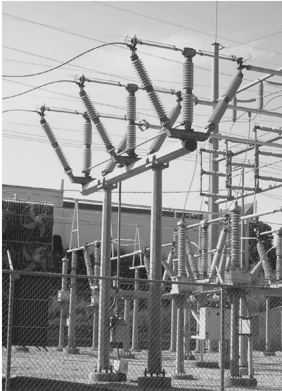
FIGURE 4.13 Double end break “Vee” (double side break “Vee”) disconnect switch.
