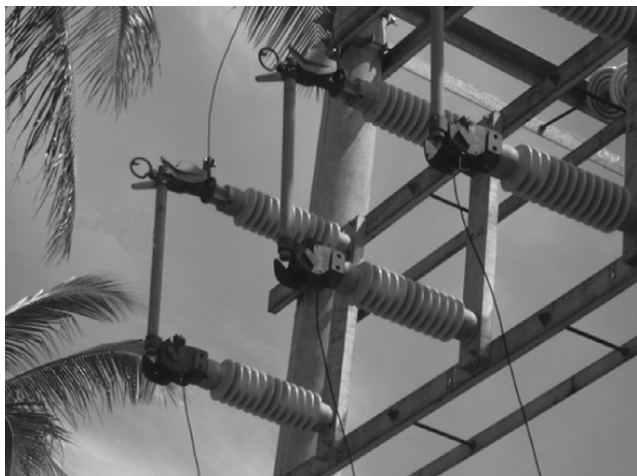
FIGURE 4.32 Vertically mounted power fuses.
