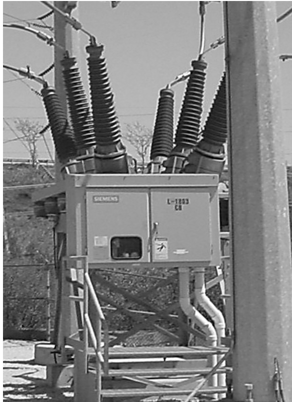
FIGURE 4.41 SF 6 gas dead tank circuit breaker.
