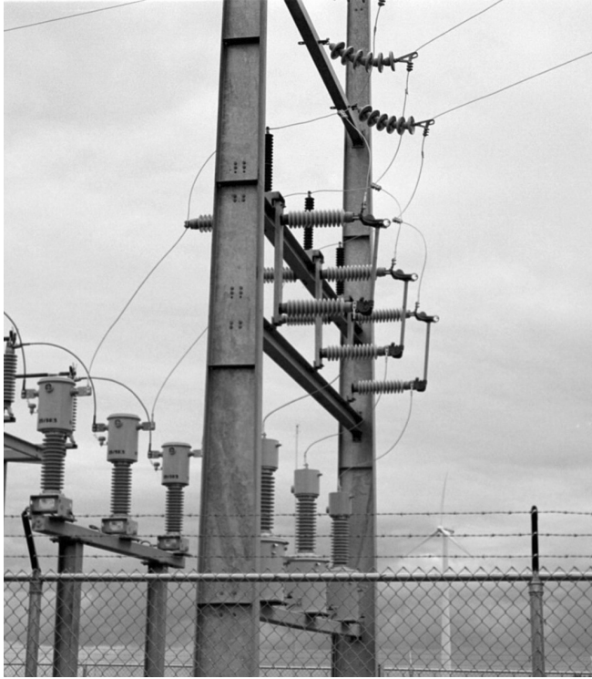
FIGURE 4.31 Incoming line structure mounted power fuses.
