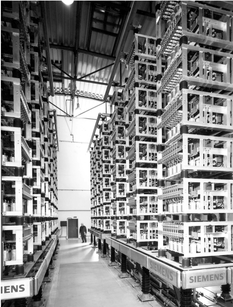
FIGURE 5.5 600 MW HVDC back-to-back converter valves. (Photo courtesy of Siemens.)
