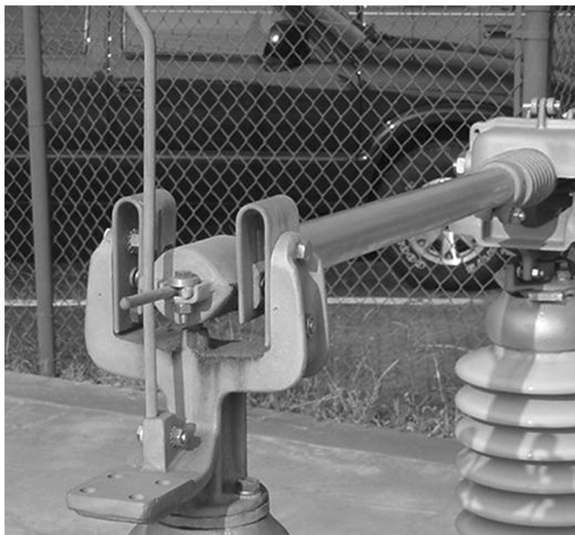
FIGURE 4.25 Arcing horns on a vertical break switch.
