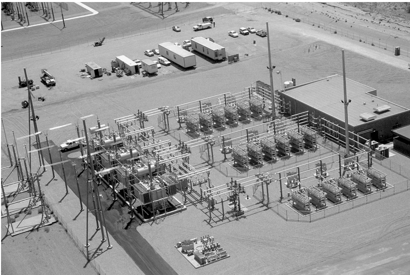
FIGURE 5.12 500 kV, 400 MVar SVC at Adelanto, California. (Photo courtesy of Siemens.)
