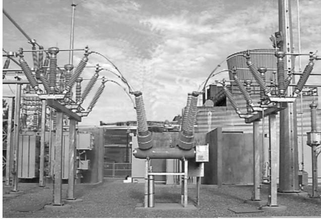
FIGURE 4.22 Double end break “Vee” disconnect switch on single horizontal member, two column structure.
