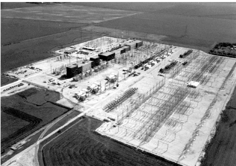
FIGURE 5.7 Dorsey terminal of the Nelson River HVDC transmission system. (Photo courtesy of Manitoba Hydro.)
