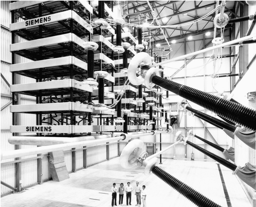
FIGURE 5.6 Valve hall of a \pm 500 kV, 1200 MW long-distance HVDC converter station. (Photo courtesy of Siemens.)
