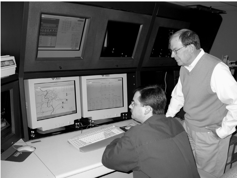
FIGURE 7.3 SCADA system dispatch center.
