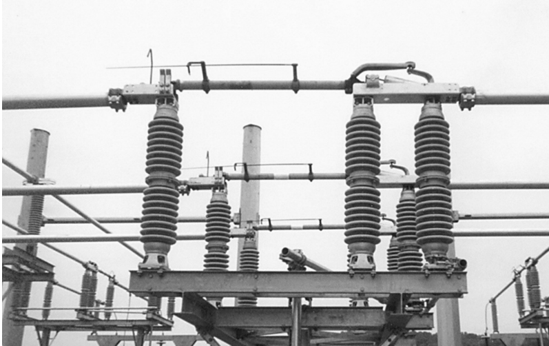
FIGURE 4.26 High-speed arcing horns on a vertical break switch.
