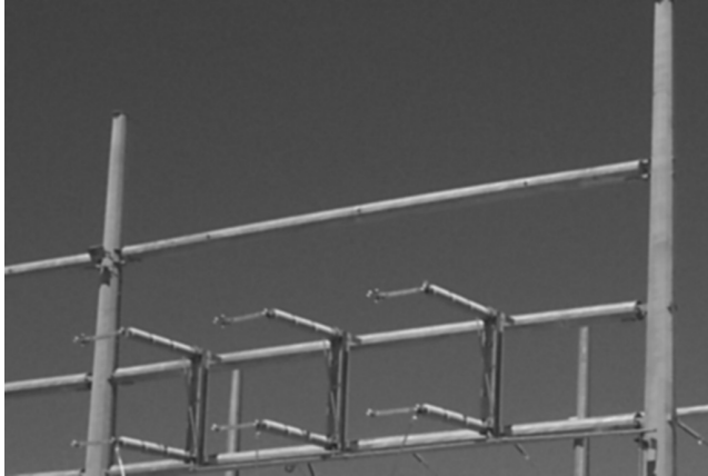
FIGURE 4.23 Vertically mounted center break disconnect switch.
