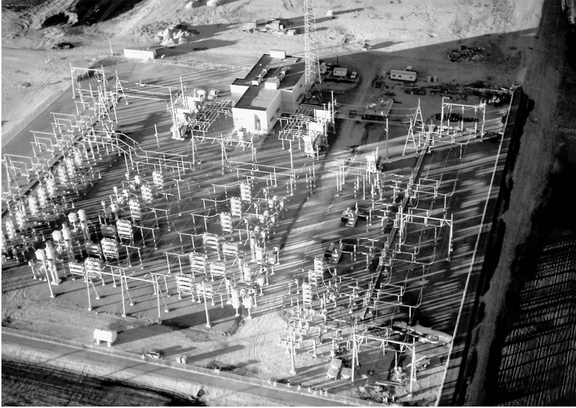
FIGURE 5.4 A 200 MW HVDC back-to-back converter station at Sidney, Nebraska. (Photo courtesy of Siemens.)
