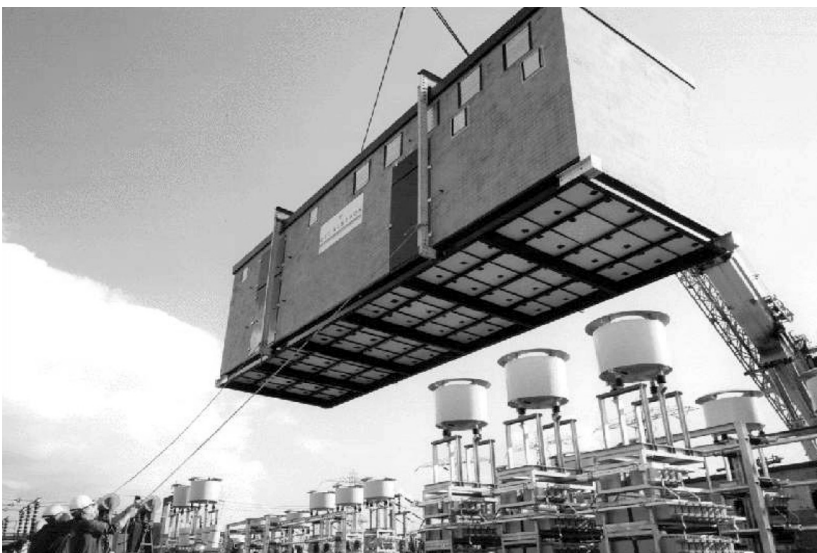
FIGURE 5.16 Static VAR compensator is relocated where the system needs it. (Photo courtesy of ALSTOM T&D Power Electronic Systems.)
