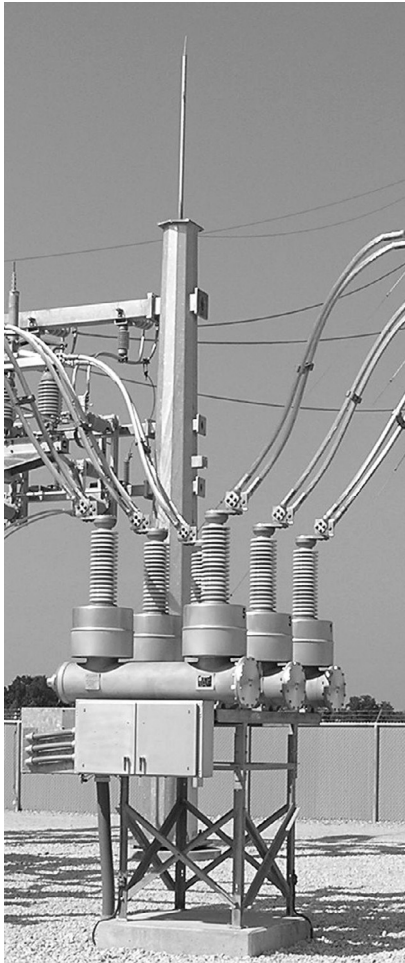
FIGURE 4.40 SF 6 gas dead tank circuit breaker.
