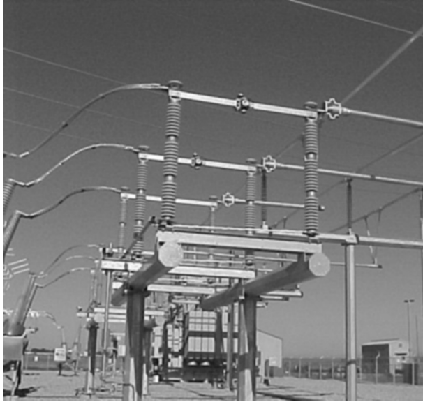
FIGURE 4.14 Center break disconnect switch.
