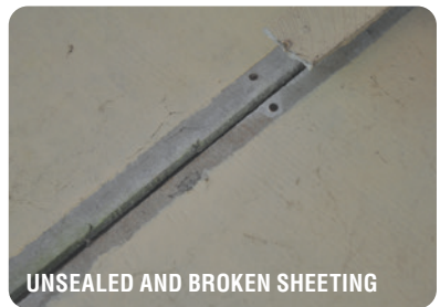
BROKEN ASBESTOS CEMENT SHEETING
