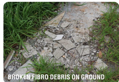
GARAGE WITH UNSEALED & BROKEN FIBRO
