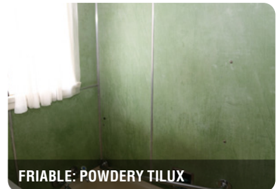
FRIABLE: UNPAINTED, EXPOSED & WEATHERED AC SHEETING
