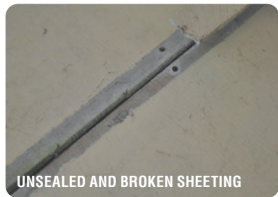
BROKEN ASBESTOS CEMENT SHEETING
