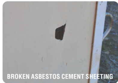
EXTERNAL PEELING PAINT
