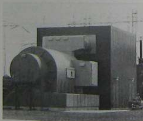
Figure 17.24b Synchronous capacitor enclosed in its steel housing containing hydrogen under pressure (300 kPa, or about 44 lbf/in 2 ). (Courtesy of Hydro-Québec)
